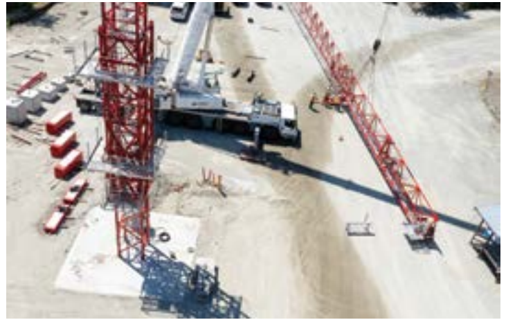
Members from both RKM and Oxford Builders working together assembling the Potain MDT 219.
