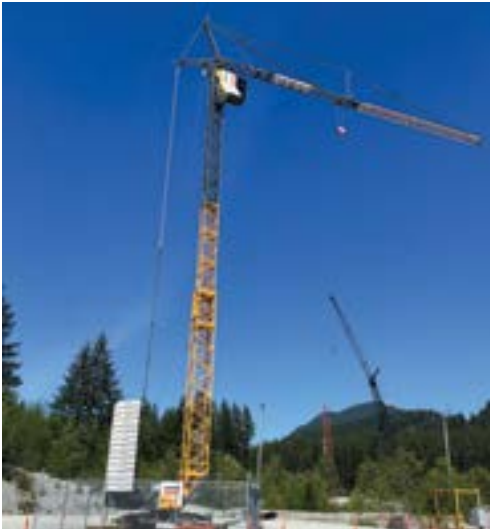
Liebherr 81K Self-Erect Tower Crane at the IUOETA training site. Thanks to Morrow Crane and their crew in assisting us with the installation of this crane.
