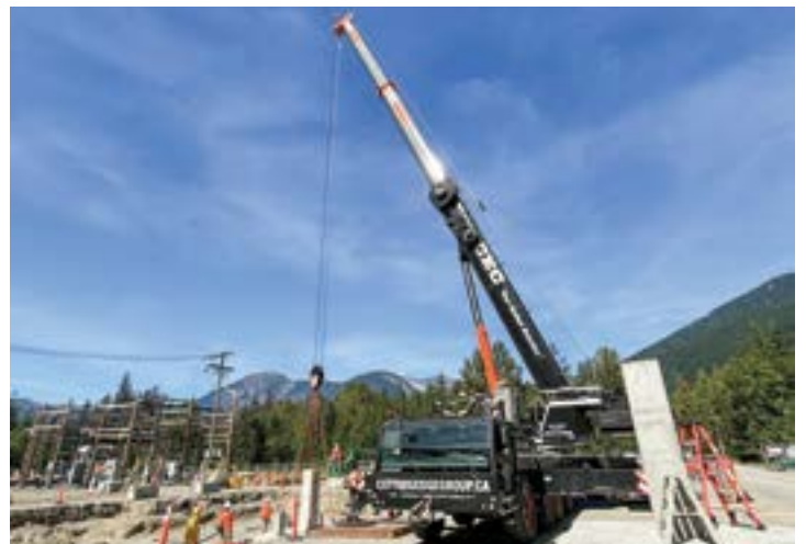
Member Ken Collins working on site in Bella Coola for Cutting Edge Crane.
