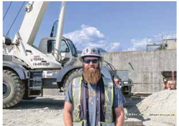
Crane Operator Warren Torris, the last standing Operating Engineer on the Second Narrows Water Tunnel Project.
