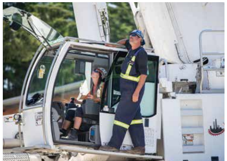
Mobile crane apprentice Karly Desjardin placing the last counter weight and last lift of the day under close supervision of Chris Brodoway.
