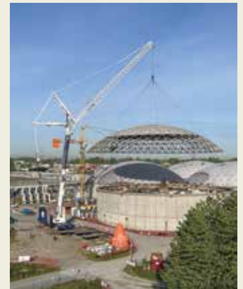
GWIL Crane members Andy Murray, Ken Grant and Matt Davis on the Liebherr LTM-1650 lifting the 68,000 lb dome off the Annacis Island Wastewater Treatment Plant.
