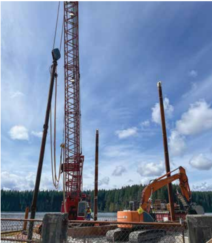
Crane operator Mike Dunlop, excavator operator Trenton Henneberg, and deckhand Brian Robertson working at the John Hart Dam.
