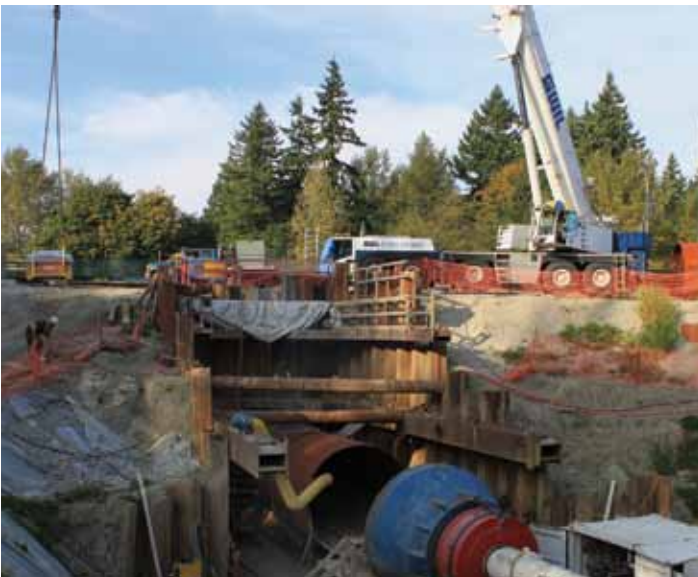
Brother Justin Mainville, working with GWIL Crane, on a site with other Local 115 members from Kamloops Augering.
