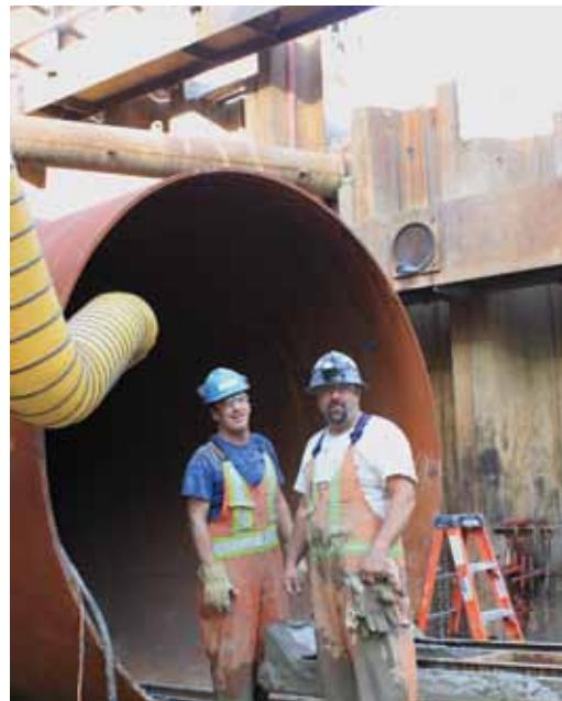
Brothers Don Gagnon and Jeff Munro standing in front of a 10' diameter steel pipe that will support a salmon-bearing stream under Highway 1 at 176th Street in Surrey.
