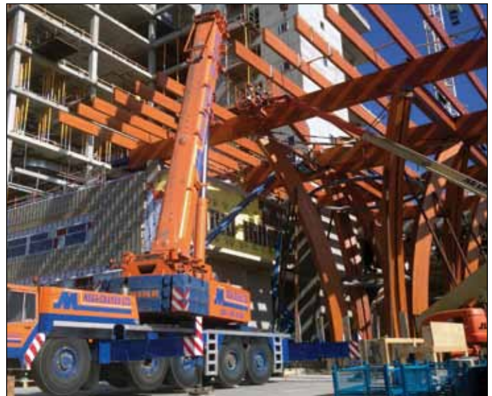
Brother Josh Vanderzwan working on the new wing of the Surrey hospital. Photo supplied by Mega Cranes
