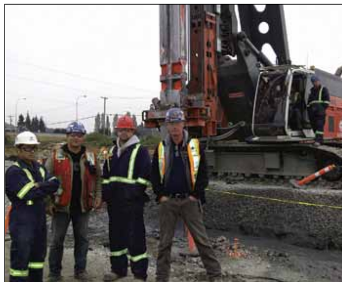
Brothers Bruce Usui, Bob Belley, Eric Sykes, Al Hurley, Brad Slyman and Carey Atchison, working with Geopac in Richmond, with the new soil-mixing machine.
